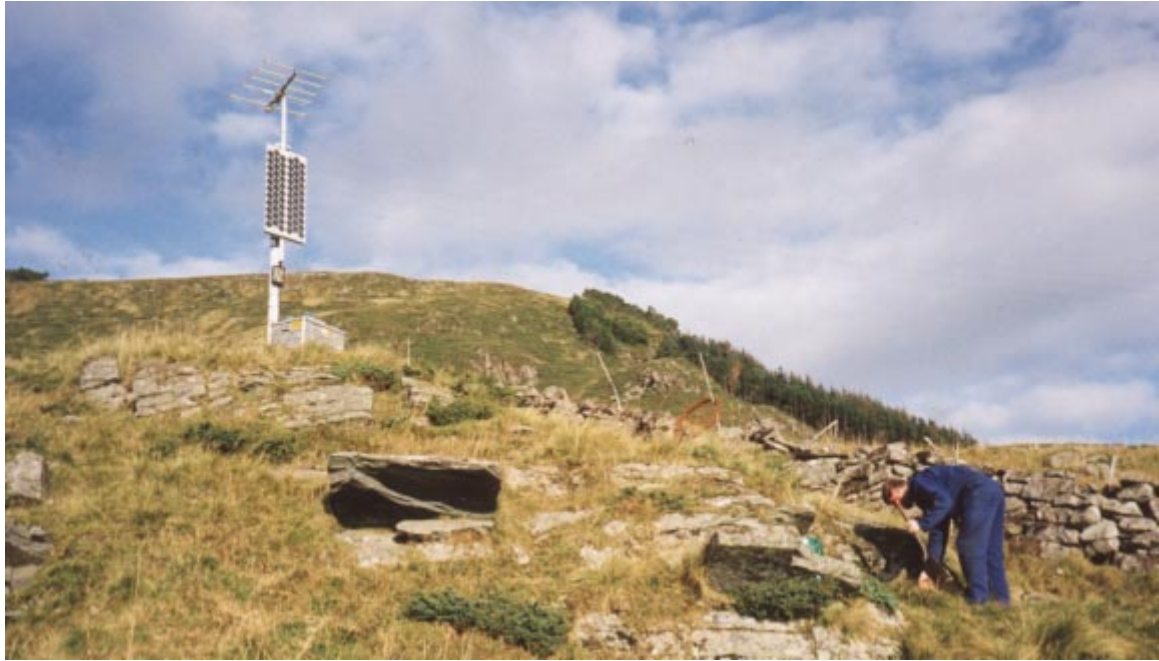
Fig. 7.1.6. The solar powered station at Drage (N2B4) on Stadlandet. The batteries are in the large box by the mast. The seismometer is under the green cover barely visible just left of K.A.Løken.
