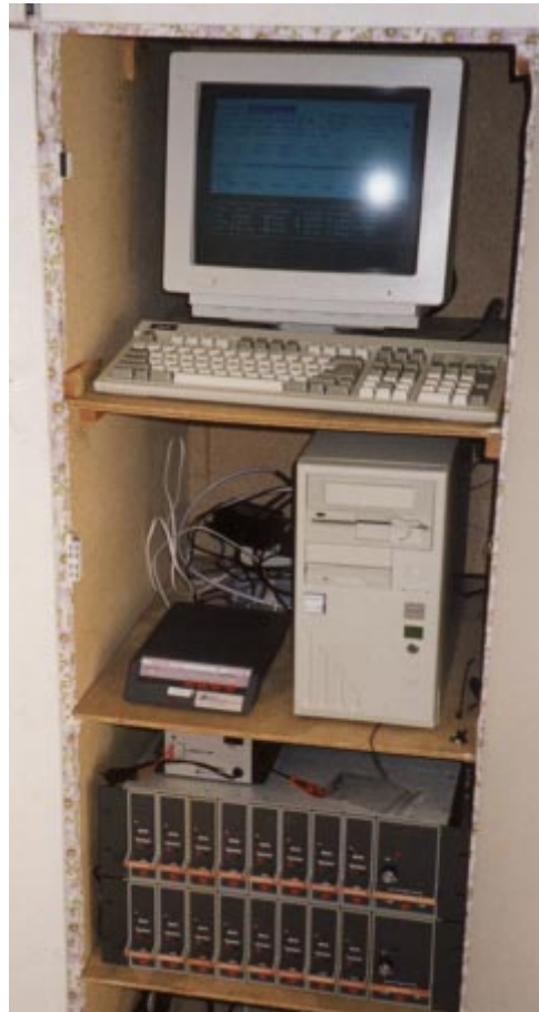
Fig. 7.1.4. The data acquisition system, Bremanger.
